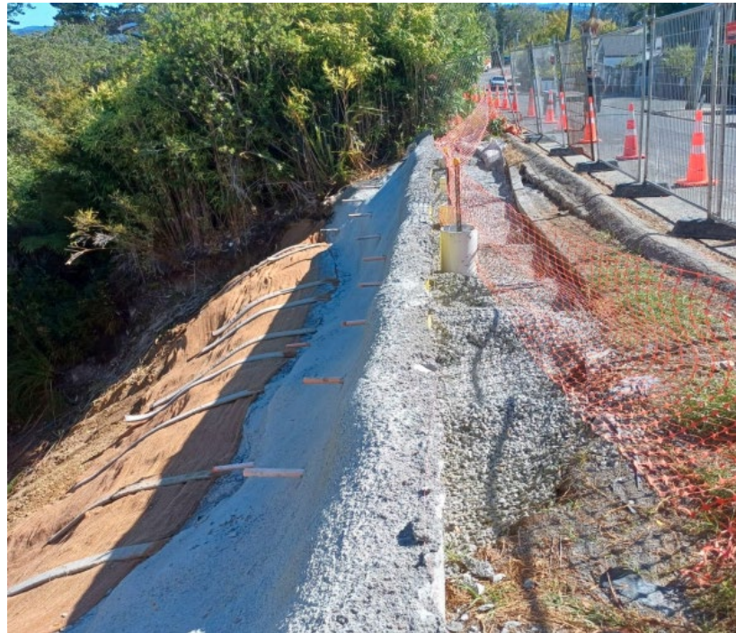
Slip on Taunton Terrace opposite #45
