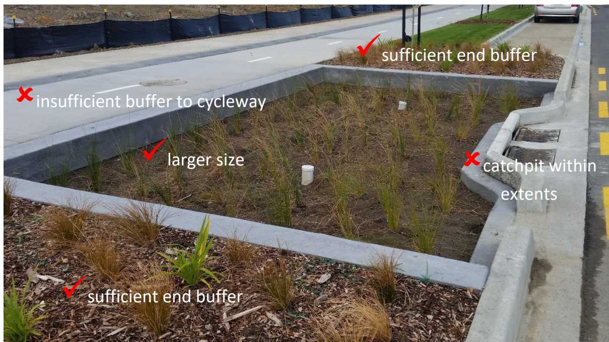
FIGURE 5-4: CONCRETE BOX ROADSIDE RAINGARDEN (1)
