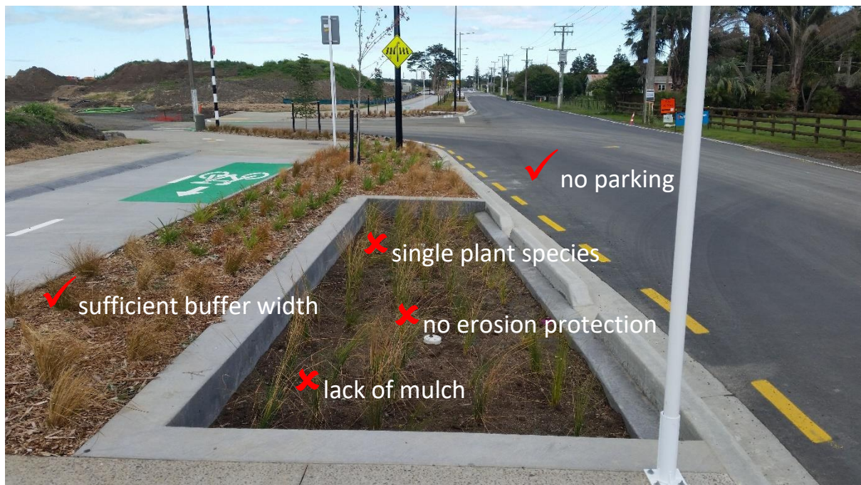
FIGURE 5-2: CUT BATTER ROADSIDE RAINGARDEN, WITH CONCRETE BORDER (2)
