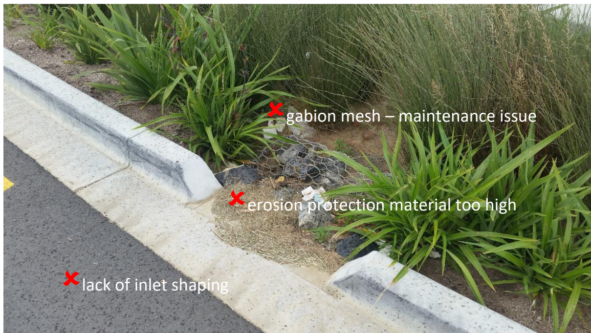
FIGURE 5-3: RAINGARDEN WITH INLET ISSUES
