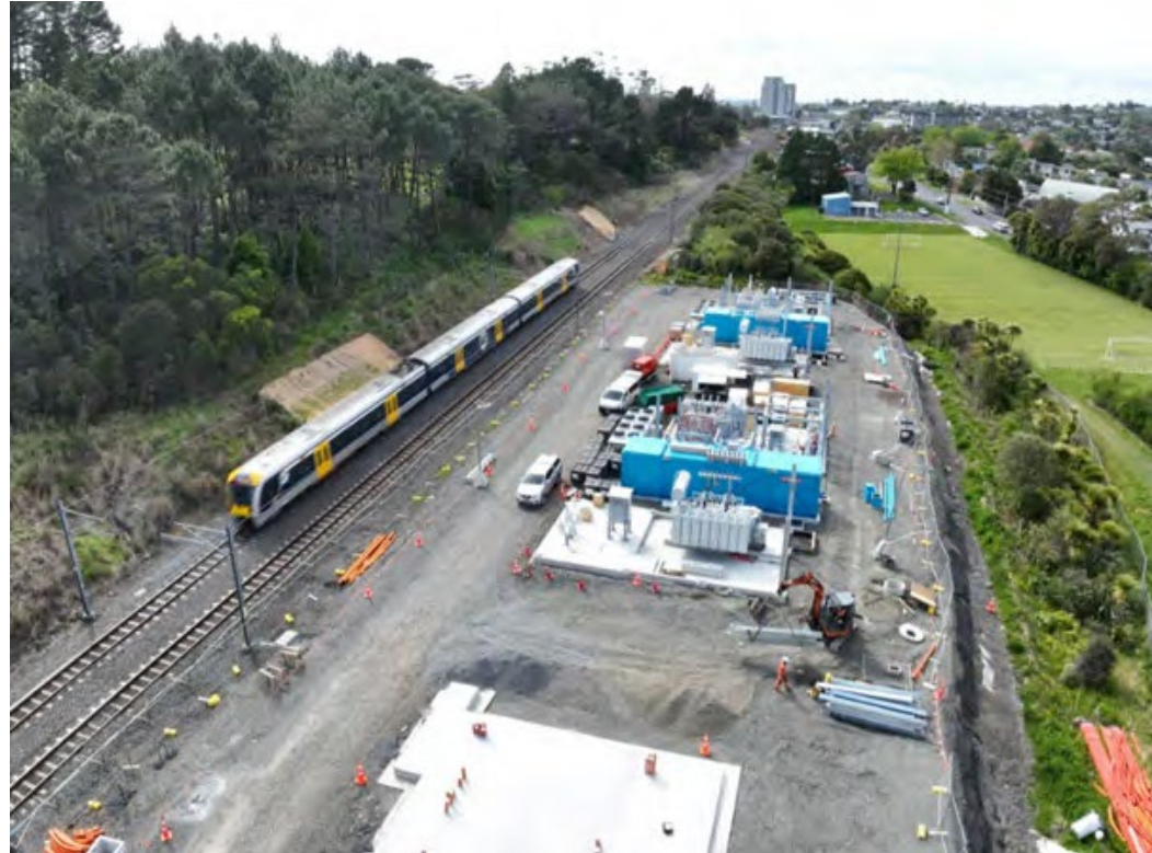
New Power Feed at Glen Eden (facing East)
