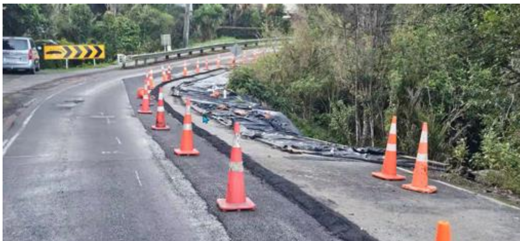
Slip site at 150 Woodlands Park Road after the relocation of the watermain.
