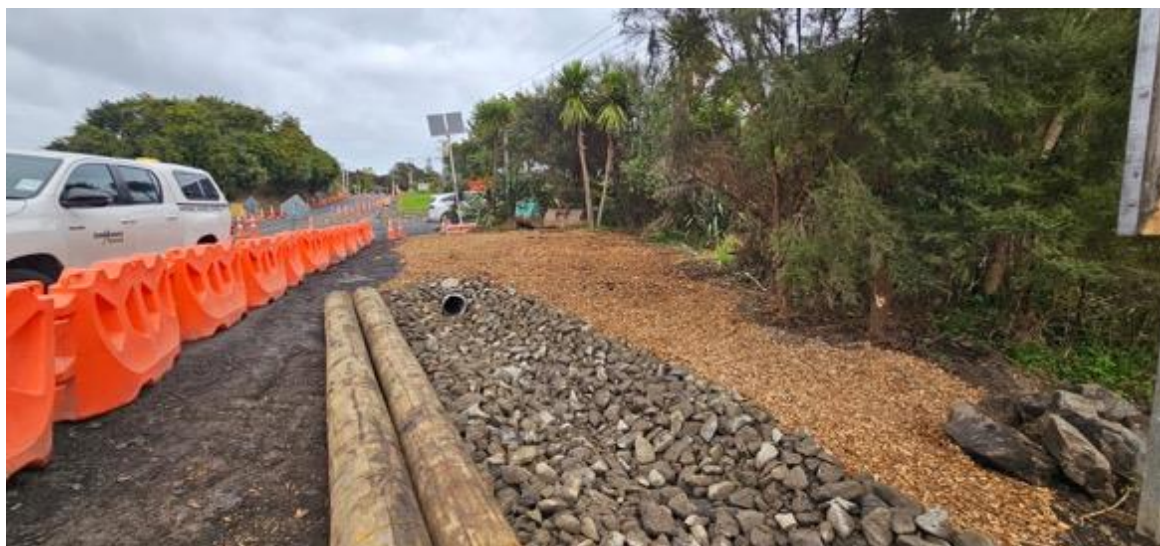
Storm water drainage
